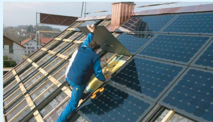
The individual MegaSlate® solar laminates are pushed beneath the upper element and fixed into the roof hooks.
