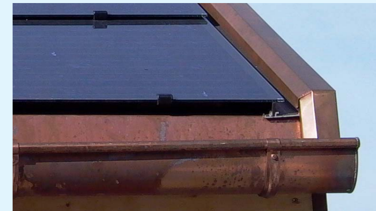
At the gutter, the ridge and the edges, standard solutions can be applied with minimal adaptation.
