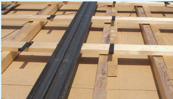
Based on the visible height of the MegaSlate® solar laminates, the battens are laid with proper spacing.
